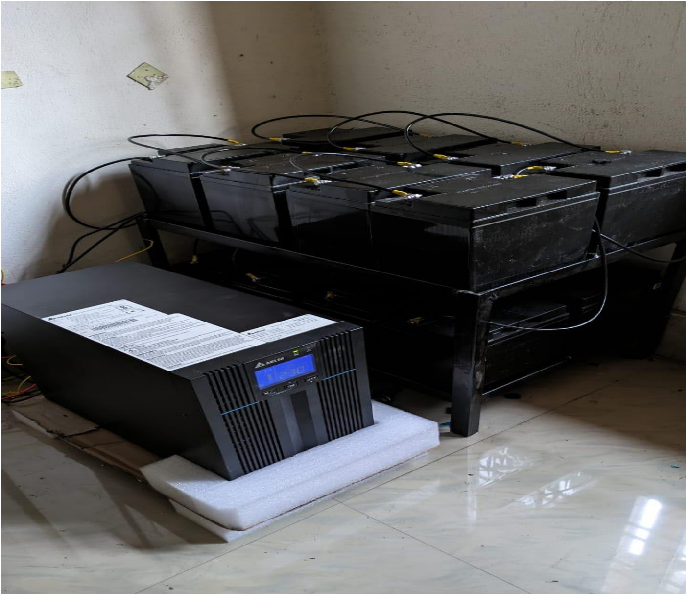
6KVA Online UPS with an Isolation Transformer
