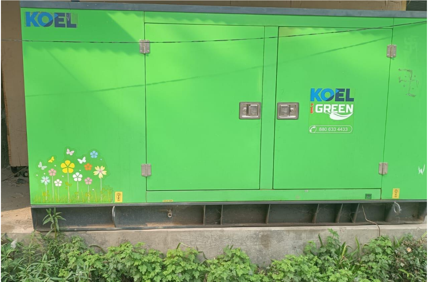
Power Generator (Substitute Energy) of College
